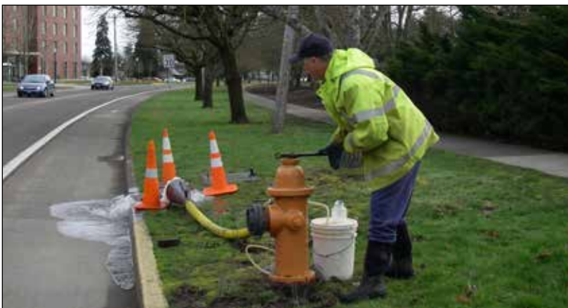
Distribution system operator Bill Ritchey flushes water lines to maintain water quality
